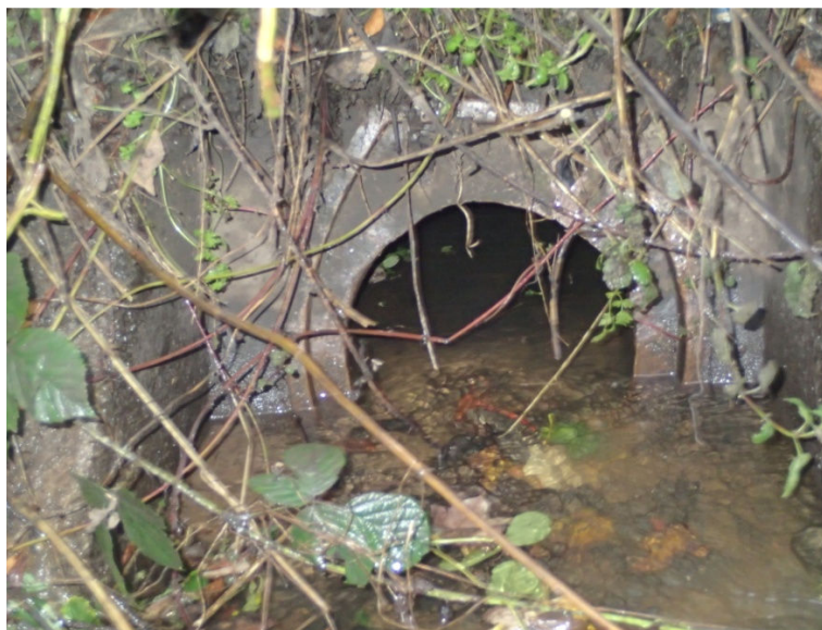
Figure 8: Outfall from Fouracres into Whinny Brook, taken 06/11/2012
